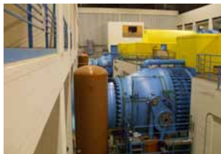
Example of a power house and turbine
